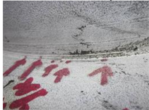
Cracks in cylinder body and flange
