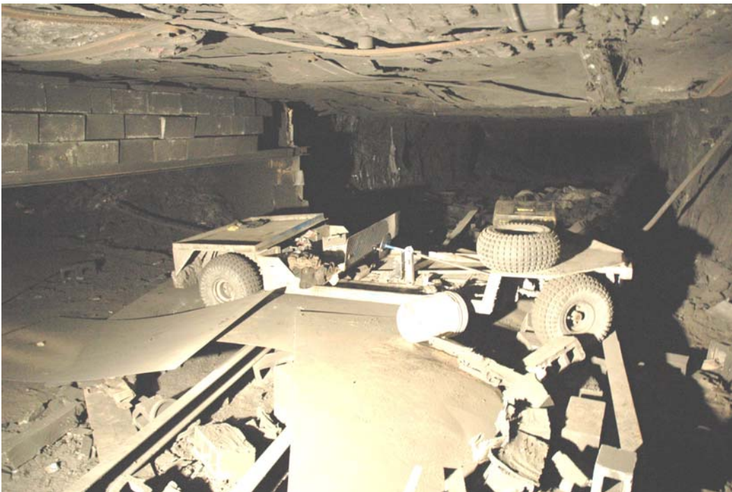
Photograph 2 - No.1 personnel carrier on damaged overcast
