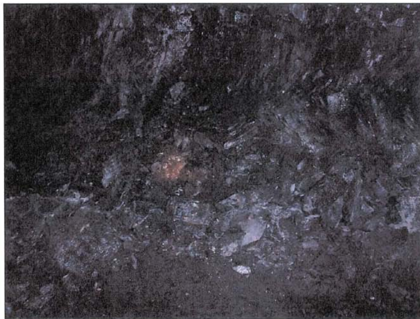
Photo 1. Rib Sloughing Near Crosscut 123 in the Entry North to the South Remnant Barrier Pillar
